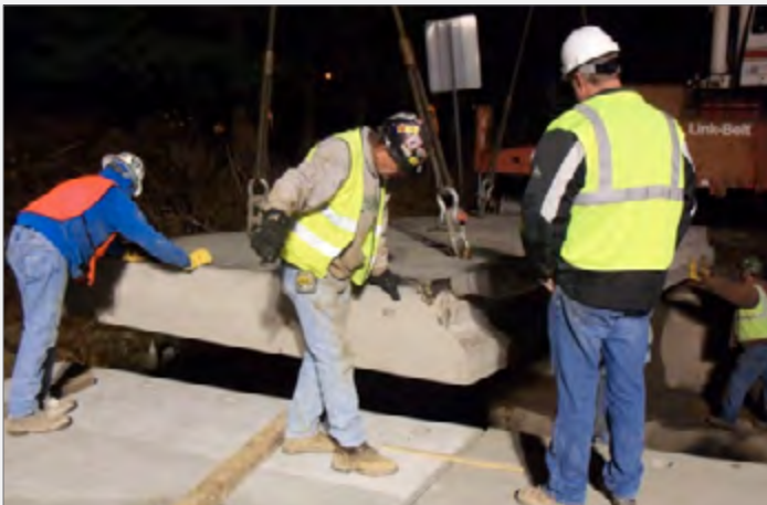
Workers install one of four bridge slabs at a job site in Harlan County.
